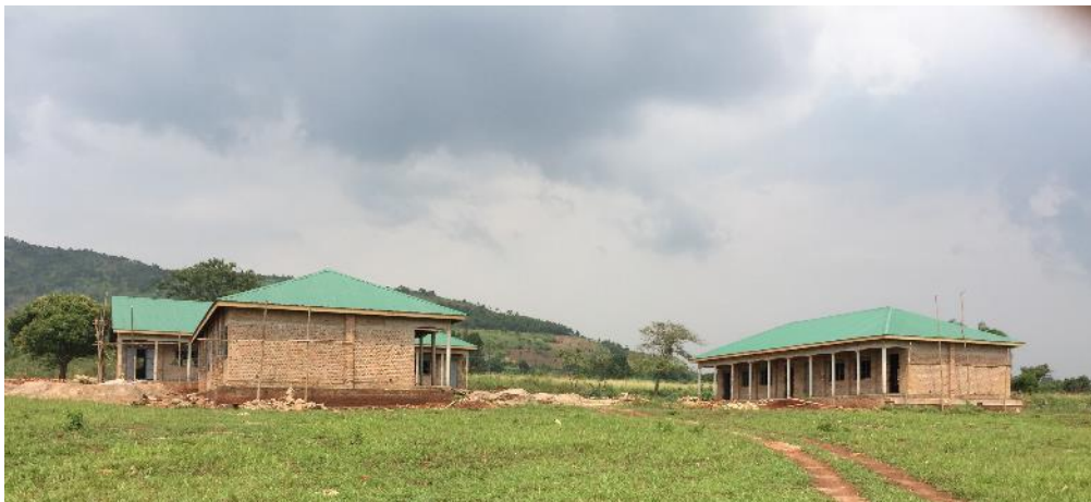
Here are the two classroom blocks with the laboratory in the background.
